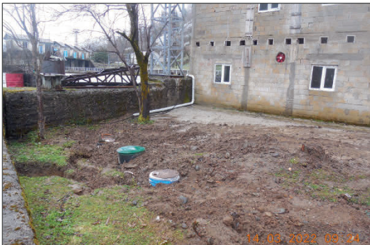
Picture 1: Biological septic tanks
