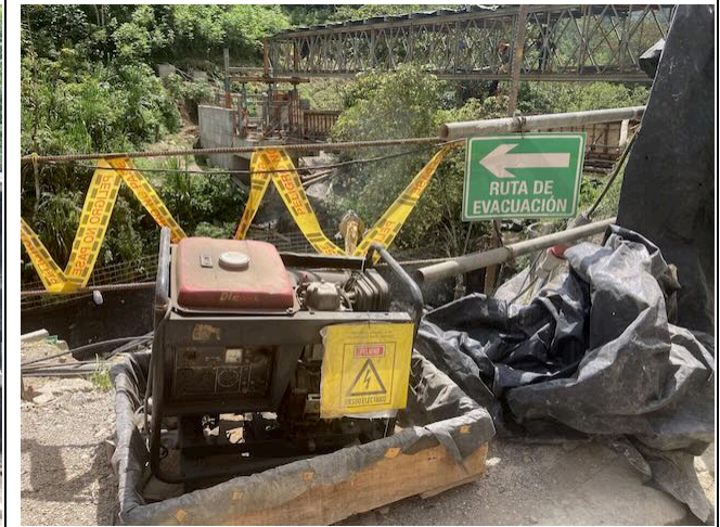
Photo 42: Construction equipment with inadequate containment 1
