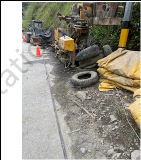
Photo 51: Inadequate waste management
