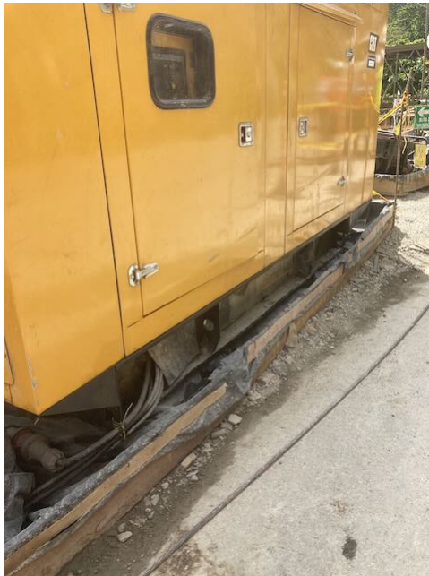
Photo 43: Construction equipment with inadequate containment 2
