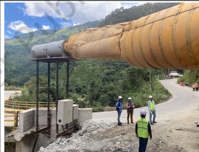
Photo 53: Ventilation at lower tunnel entrance
