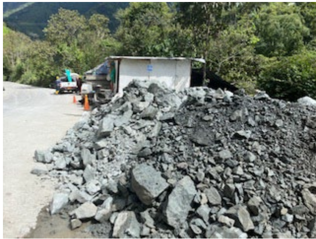
Photo 40: Inadequate containment of excavated material from tunnel
