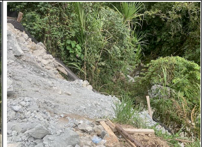
Photo 18: Temporary spoil deposit at upper tunnel portal, at risk of sliding into river
