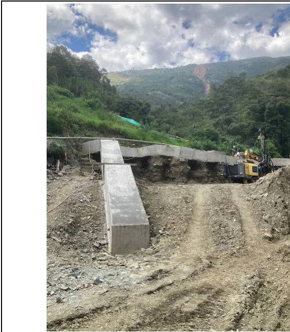
Photo 49: Containment wall between future powerhouse below and spoil deposit from road construction above
